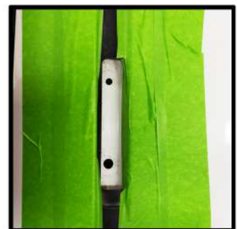
View of bottom hole drilled, be sure to clean any shavings away that fell thru while drilling.
