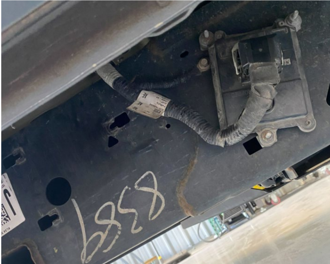
Figure 22: Correct Relocation of Fuel Control Box
