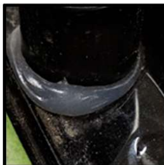
Before placing the spacers down apply a liberal amount of sealant to ensure a water tight seal
