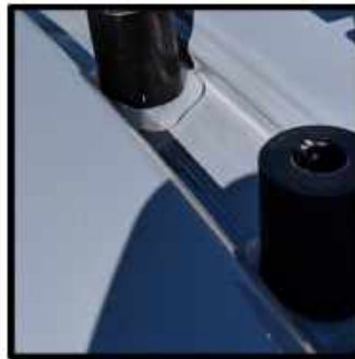
APPLY A LIBERAL AMOUNT OF SILICON OVER THE HOLES AND THEN PLACE THE SPACERS ON TOP TO INSURE A WATER TIGHT SEAL
