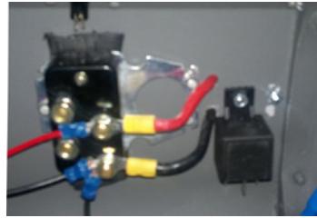
UNCOVERED-Location of relay
