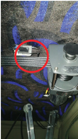
Location of Limit Switch near the winch motor
