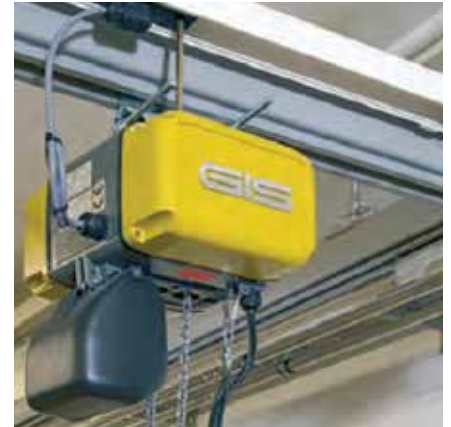
ENCLOSED CONDUCTOR LINE
