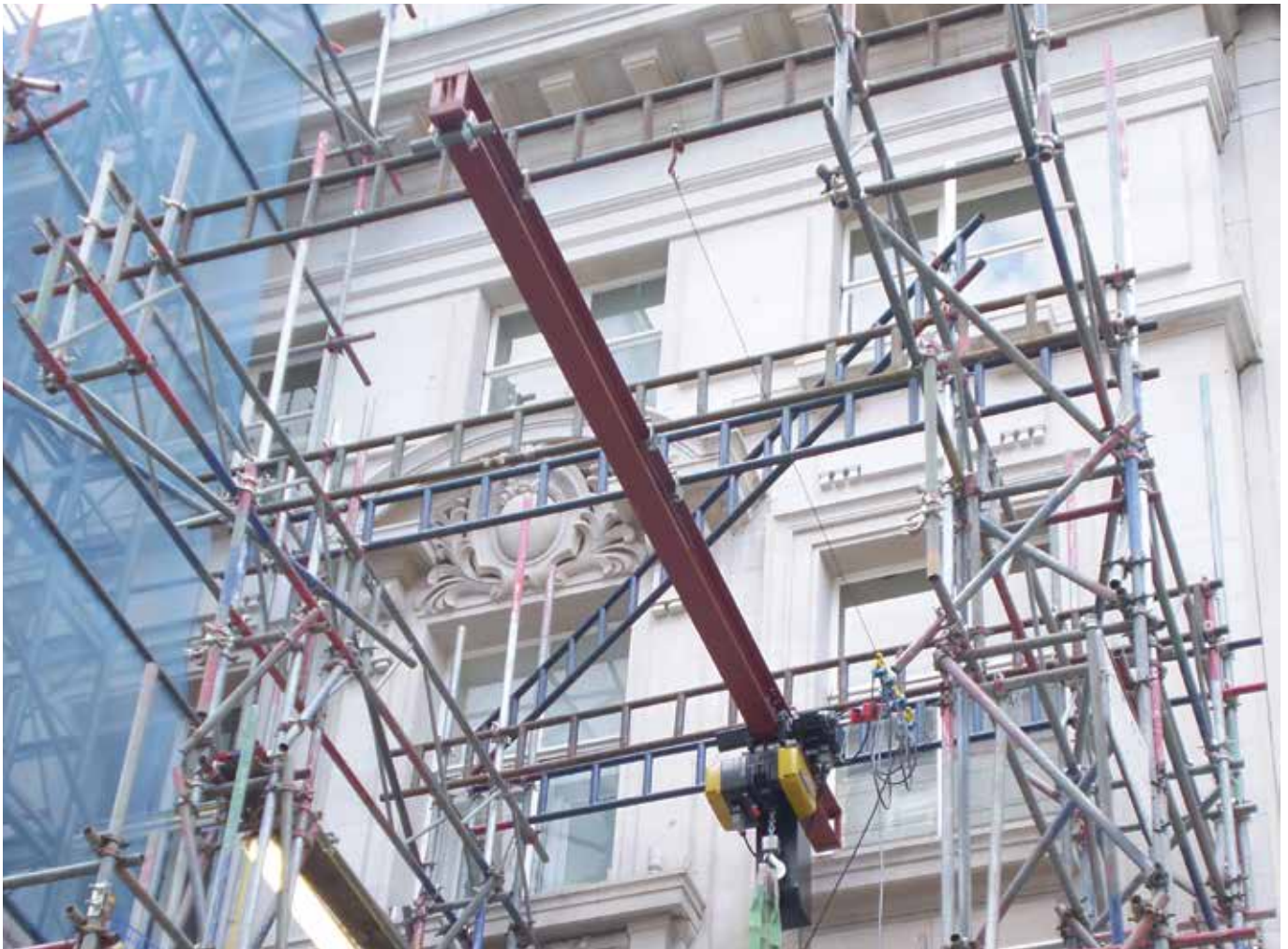
GIS HOIST ON A GANTRY BEAM APPLICATION, SUSPENDED FROM SCAFFOLD
