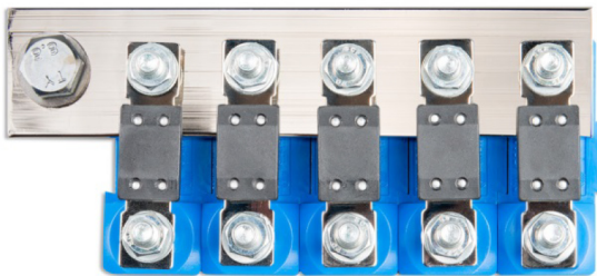
Stacked fuse holders with 5-position high current bus bar (copper 40 x 5 mm)
