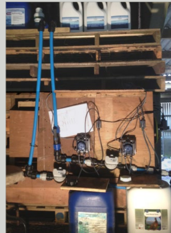
Customer's two Stenner Pumps in use dosing Intra Hydrocare and Quill Boost
