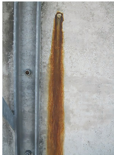
Figure 5.4 Rust staining that may indicate corroding reinforcement (or a metal fixing) (courtesy CH2M Hill, with permission from the Environment Agency)
