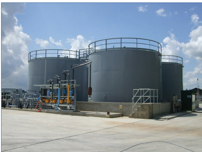
Figure 9.3 A vertically cylindrical welded-steel tank (courtesy M.C. Integ Ltd)
