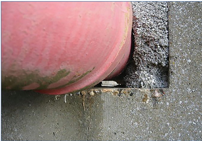
Note the pipe is bearing on the formed hole such that the infill concrete or mortar beneath will not form an adequate seal. In addition there is no puddle flange on the pipe.
