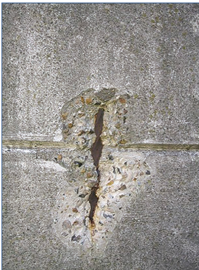
Figure 5.3 Spalling of concrete over corroding reinforced bar, where cover is reduced by groove feature (courtesy CH2M Hill, with permission from the Environment Agency)
