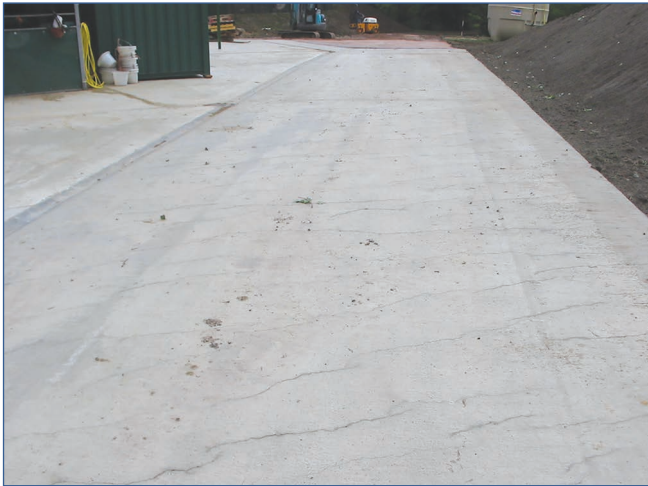
Figure 7.6 Plastic shrinkage cracks (courtesy Concrete Society)
