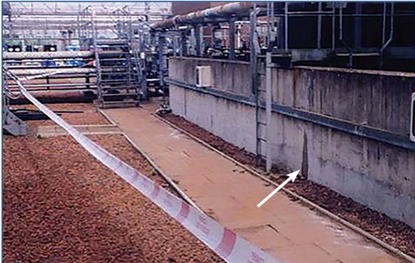
Figure 5.2 Arrow shows leaking crack in a bund wall (courtesy CH2M Hill, with permission from the Environment Agency)
