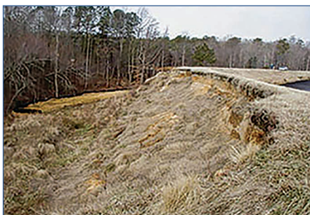
Figure 5.5 Slumping of earth embankment
