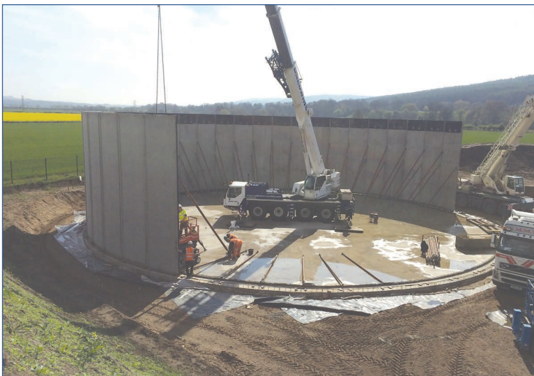
Figure 9.4 A precast concrete segmental tank construction (vertically multi-straked tank) (courtesy A-Consult Ltd)
