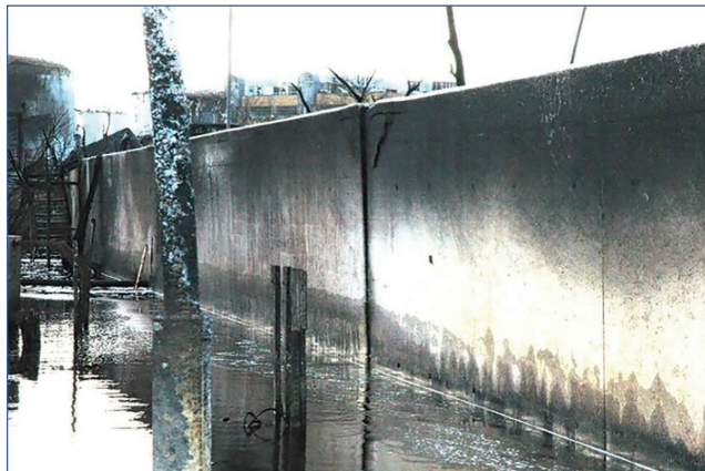
Figure 5.12 A joint that has failed due to thermal expansion because of inadequate dowel provision across the joint. Note also that the tie bolt holes at the foot of the wall also leaked during the incident (courtesy CH2M Hill, with permission from the Environment Agency)
