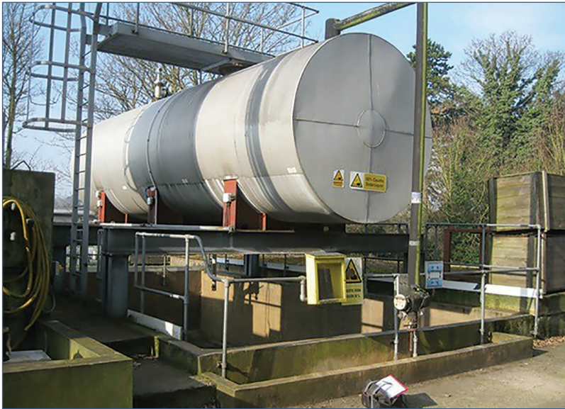
Figure 6.4 Example of installation vulnerable to jetting of fuels over the bund wall (courtesy CH2M Hill, with permission from the Environment Agency)
