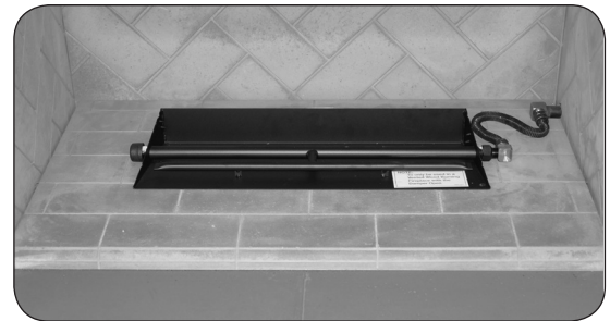
Fig. 10-2 Center burner in fireplace
