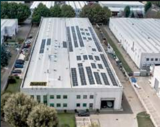
Clean energy production from solar panels
