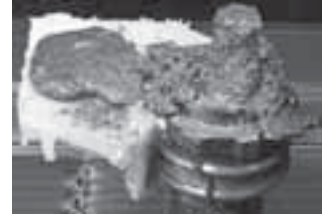
Figure 5 – Picture of a melted battery terminal
