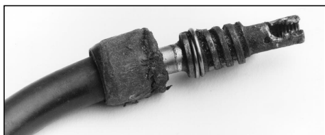
Figure 12 Spatter Damaged Swan Neck
