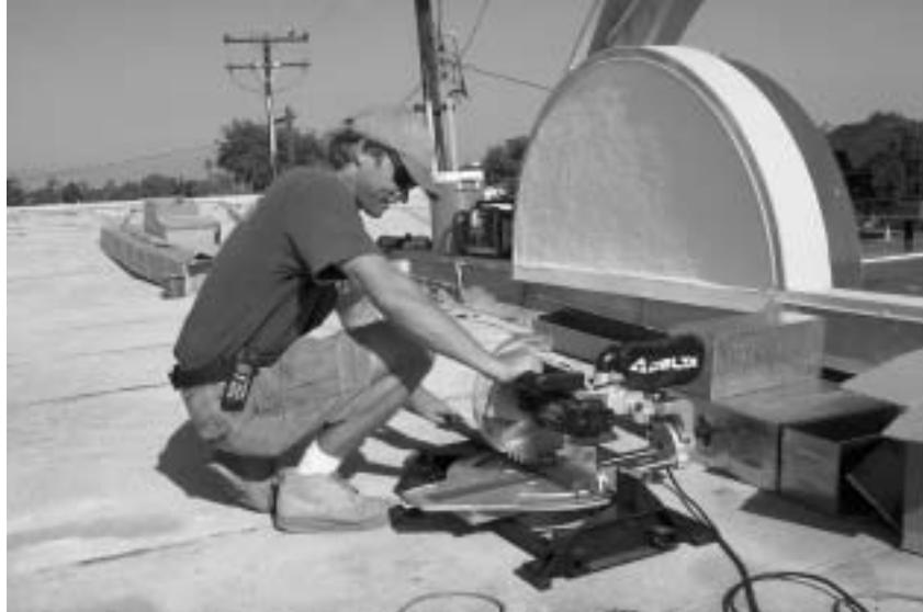
Cutting a BriteStripe section to length to fit the end of the building Figure 13
