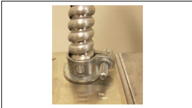
Figure 6. Non-Ferrous Fitting on Junction Box (not user serviceable)
