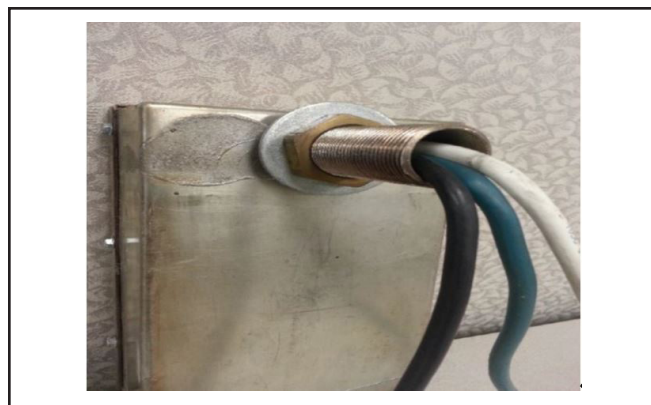
Figure 12. EMI Facility RF Filter
