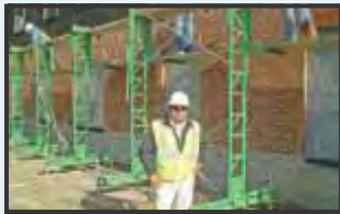
"We can move 105 feet of Workhorse to the next wall in 20 minutes." Carlos Reyes, WT Construction, New Orleans
