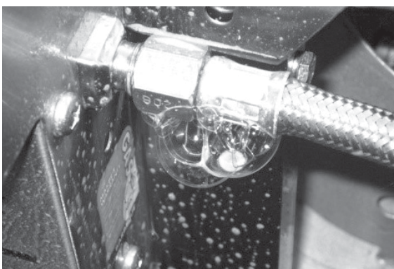
Photo of what a typical leak looks like.
