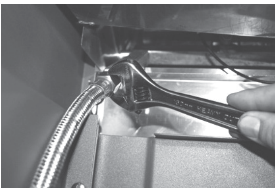
BBQ inlet connection.
