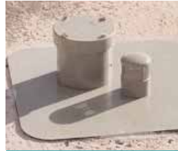
Vent cowl fitted to the top of a concrete tank to ensure air can enter the tank allowing the water to breathe.
