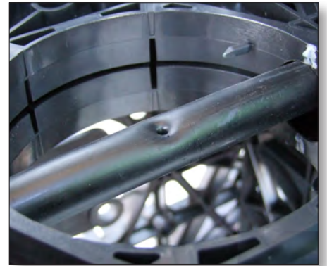
Punctured poly irrigation pipe
