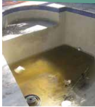
Stagnant pooling water
