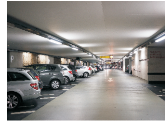
Parking lot lighting
