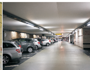
Parking lot lighting
