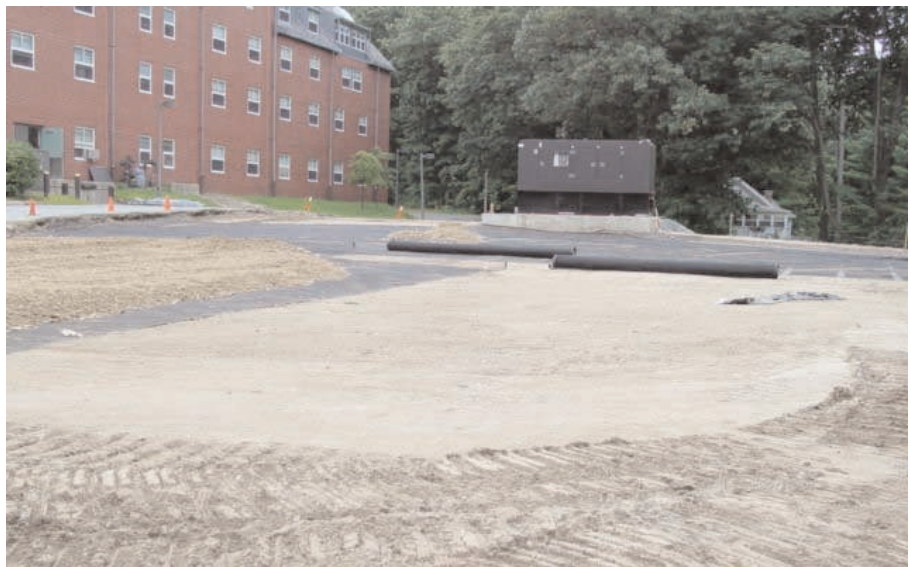
Mirafi® BXG11 was installed for the parking area and Mirafi® HP370 was used to reinforce the top perimeter of the slope.
