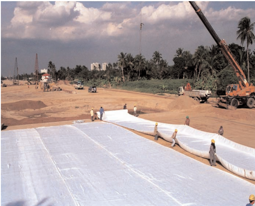
Mirafi® PET1000 was installed across the pile caps. Embankment fill was placed on top.
