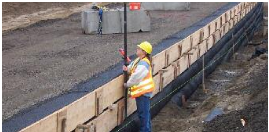
Wood forms being used to achieve compaction at the face of the wall.
