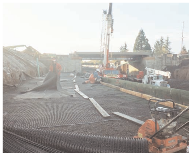
The construction of the MSE walls along the southern portion of the new roadway.
