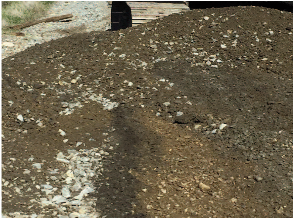
Contaminated rail ballast: The dark material is topsoil that has migrated into ballast. The lighter area is sub-ballast, which has migrated into ballast.
