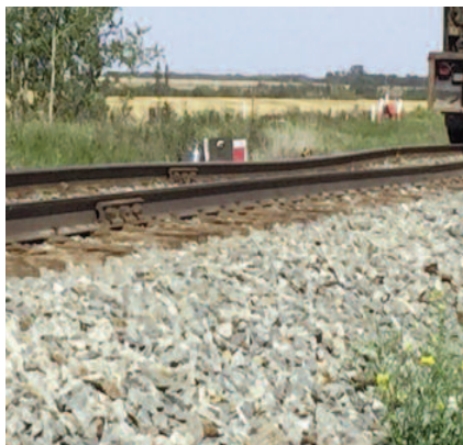
Unrepared track section with cross level variation due to settlement issues.
