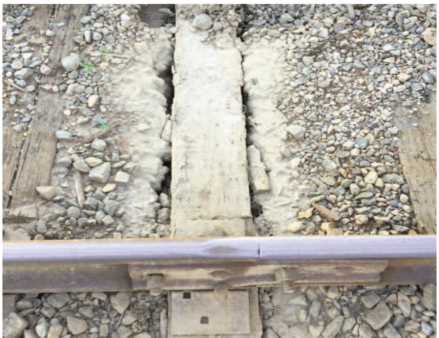
Evidence of mud pumping and ballast contamination prior to repair.
