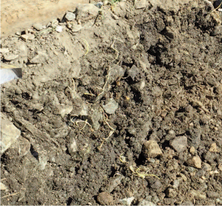
Ballast contamination and moisture enough to support plants and root systems.
