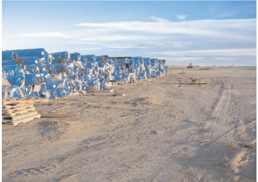
Protective wrapping was used to prevent UV degradation while the geotextiles were stored on the site.
