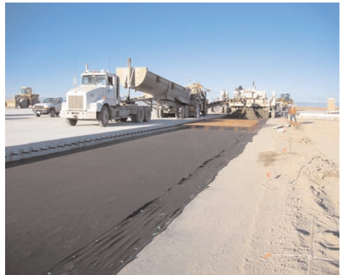
17 inches of concrete pavement was placed over the Mirafi® MPV600 and CTB subbase.
