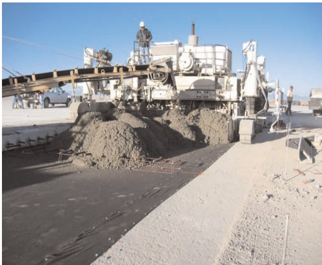
The Mirafi® MPV600 bond breaker paving fabric was placed between concrete pavement and subbase.
