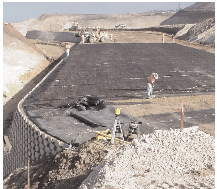
The contractor was able to install 5,000 yds 2 of Miragrid® geogrids a day.
