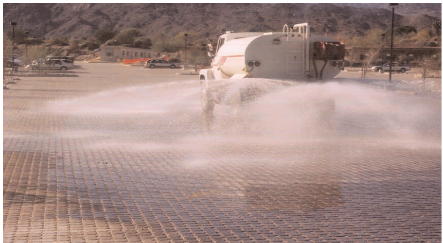
The porous pavement system is a durable and environmentally friendly design. A water truck unloads 1800 gallons (8,183 L) to prove the infiltration capacity.
