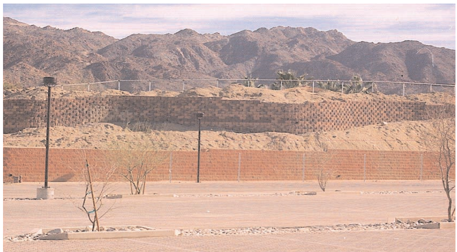
The retaining wall heights varied from 8ft. to 12ft. and also utilized two tiered designs to save costs.
