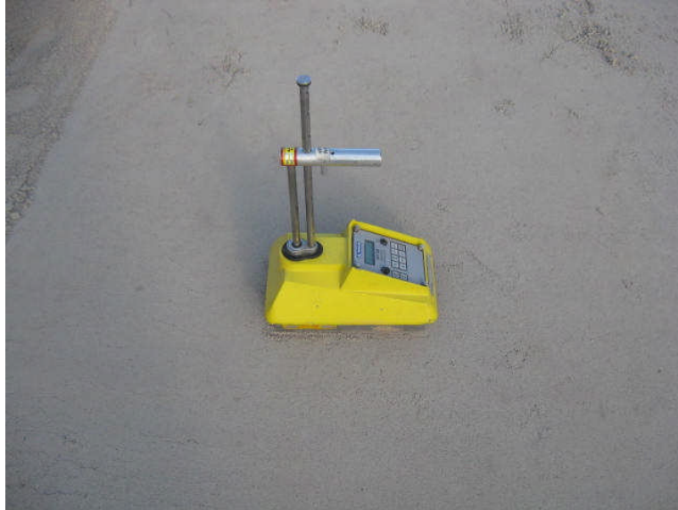
Figure D-9. The density of the compacted soil is measured with a nuclear density gauge.
