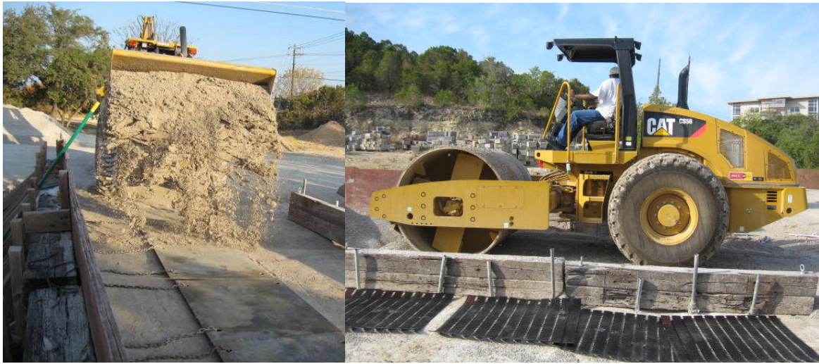
Figure D-7. Lifting Plates positioned between ties and covered with first lift of compacted soil/aggregate.
