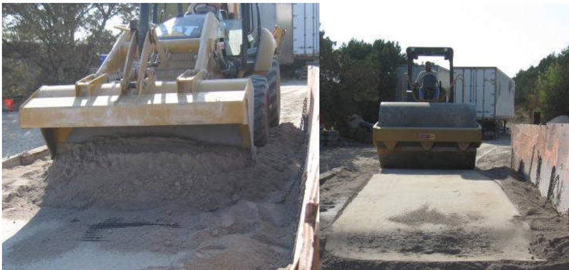
Figure D-8. Grid positioned over compacted base and covered. Cover soil/aggregate is uniformly spread and compacted using field-scale equipment and procedures.
