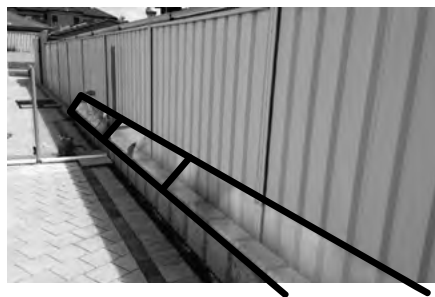
Oscillot® installation with rigid polycarbonate blocking off ledge on raised retaining wall eliminating it as a potential platform.
