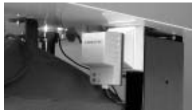
Control panel with LEDs
