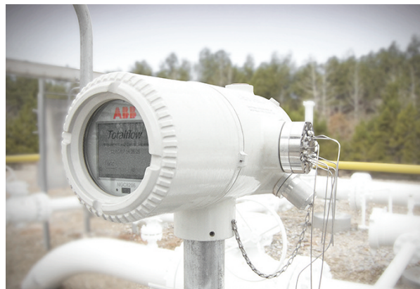
An ABB NGC 8206 gas chromatograph on a gas pipeline in Louisiana
