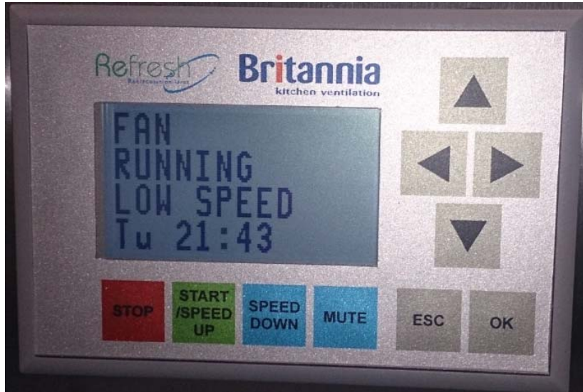
Refresh Control Panel
