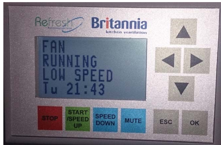
Refresh Control Panel
