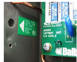
Ground in System Enclosure
