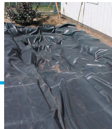
Installing the liner... Be sure to leave a few extra inches of liner in the pond. These small wrinkles will be covered by the stone and will allow the liner to stretch into place when the pond is filled with water.
