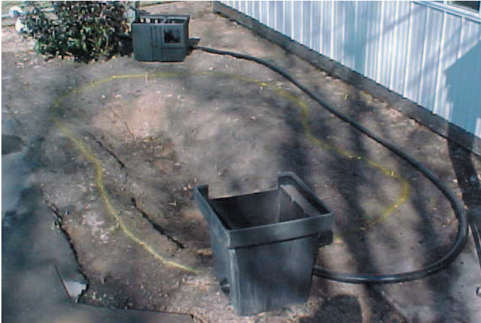
Here we are redoing a small pond in front of a business. The previous pond did not have a skimmer or Aquafalls filter. The owners wanted the pond larger and a stream added. Note the shape has been painted and skimmer, filter and pipe are in position.
