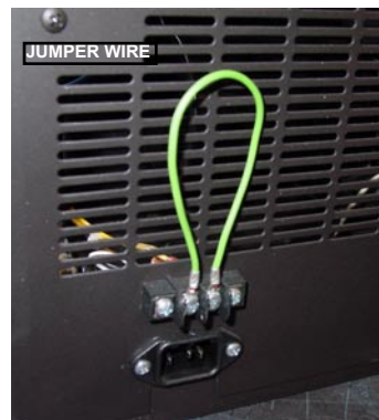
THERMOSTAT BLOCK WITH A JUMPER WIRE ATTACHED.
