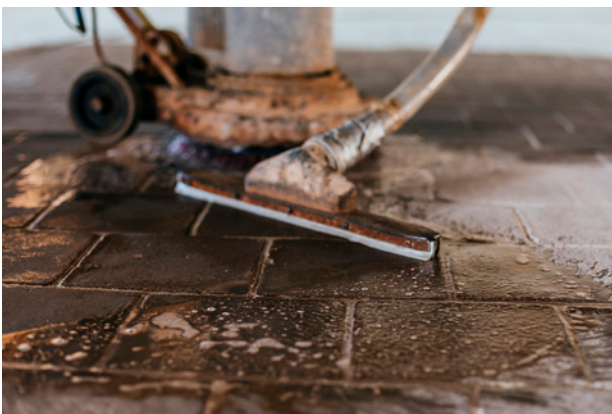
1.3. Next, we carry out a quick drying with a liquid vacuum, in case the floor is not clean enough, the process will have to be repeated small surfaces .
