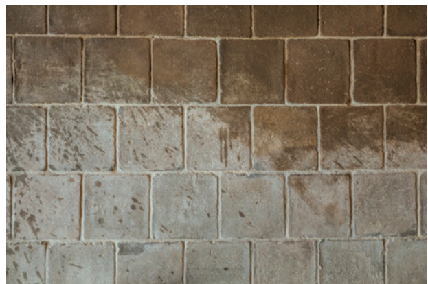
1.4. Difference between clean area of the floor (upper part of the photograph) and area to be cleaned (lower part of the photograph).
