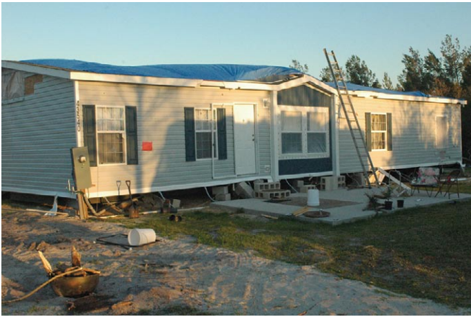
This home, which was secured with ground anchors, moved enough to allow it to fall from its supporting piers.
