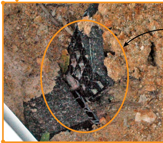
Fractured ABS stabilizer plate
