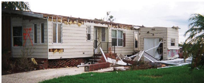
Damage to new manufactured home resulting from improper carport attachment.
