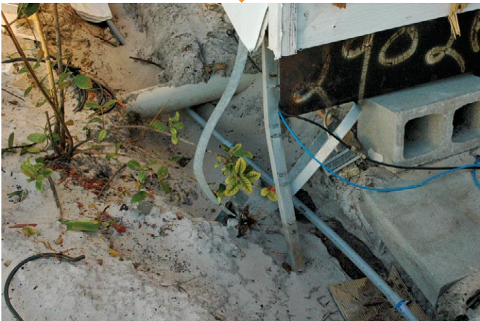
When the home shifted, anchor straps became loose.
