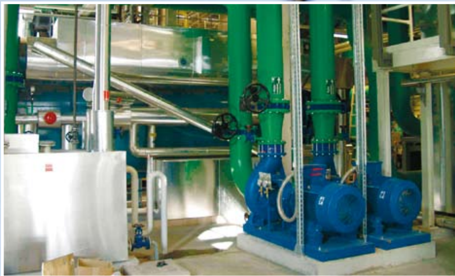
These cool water pumps at a printworks are used to ensure humidity is kept at the desired level.
