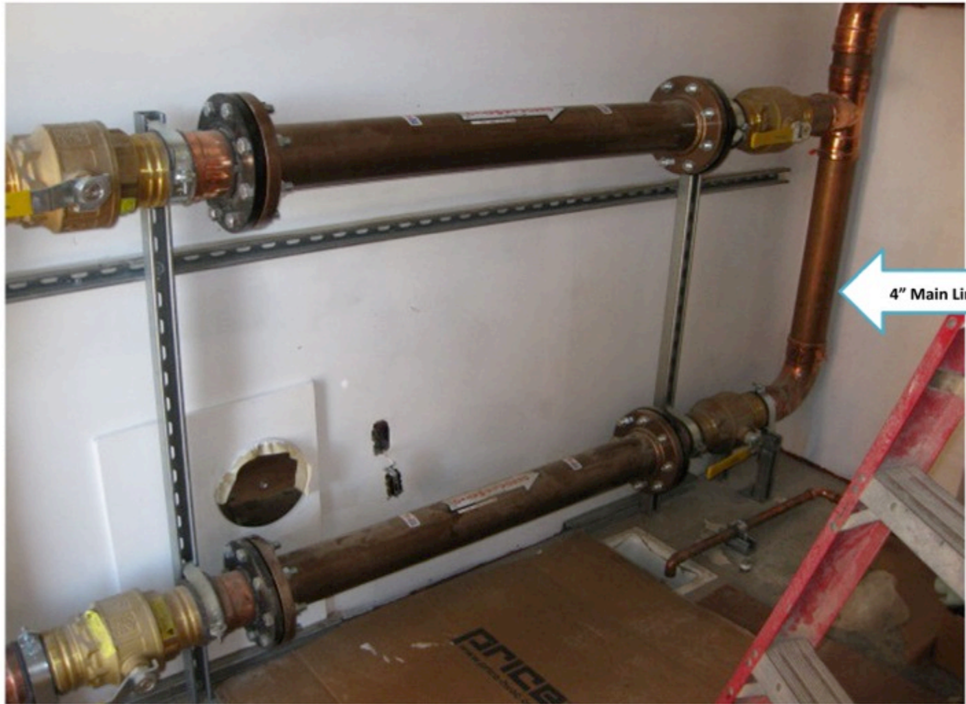
Two 200 gpm, 4" flanged Descal-A-Matic Units installed in parallel, treating the 4" main water supply line to the 93,000 sq.ft. Eisenhower Medical Center
