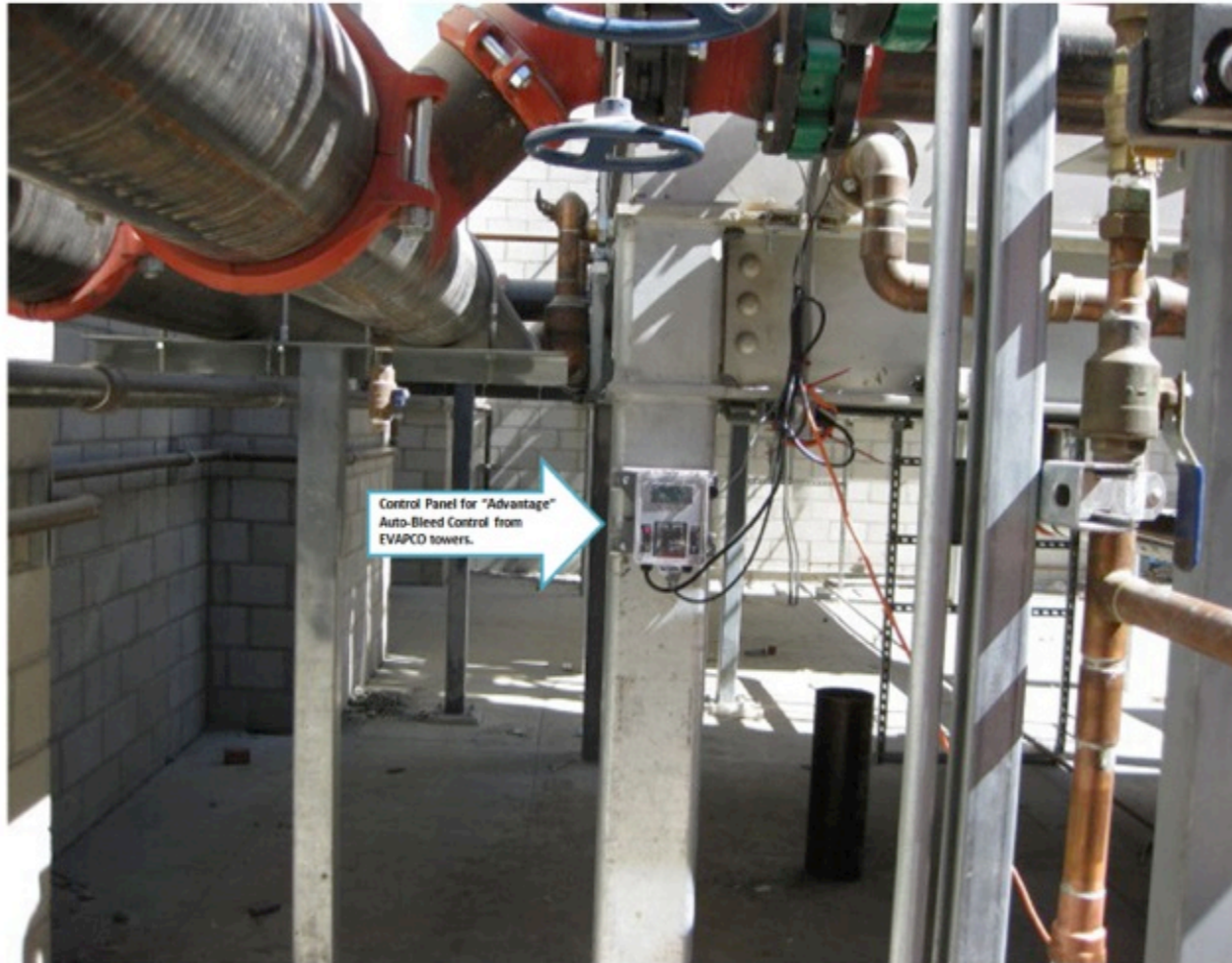
"Advantage" Auto Bleed Control from 2 EVAPCO Cooling Towers. Saves this client TONS of money in water savings.
