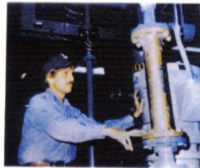
Columbia Center Building Maintenance Engineer and Descal-A-Matic® unit
