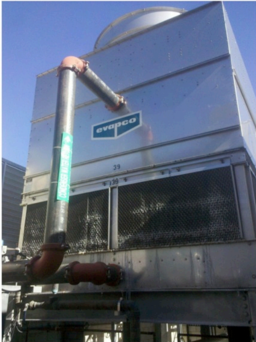
One of the two EVAPCO Cooling Towers at the Eisenhower. 93,000 sq.ft. Medical Facility in La Quinta in So. California.
