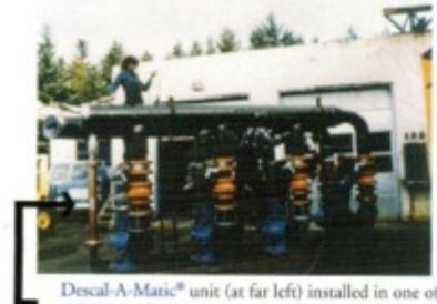
Descal-A-Matic® unit (at far left) installed in one of the many hydronic systems at Columbia Center
