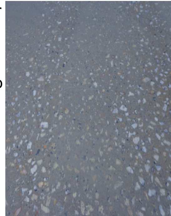
Just grouted concrete ready to start with resin bond discs when completely dry.
