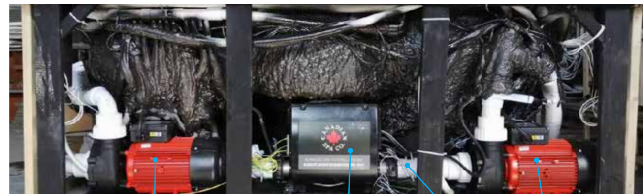
Pump Control pack Heater Pump
