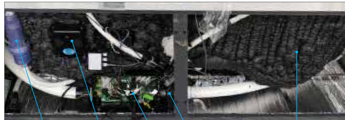
Ozone Mixing Chamber Ozone Generator Control pack Heater Black out insulation
