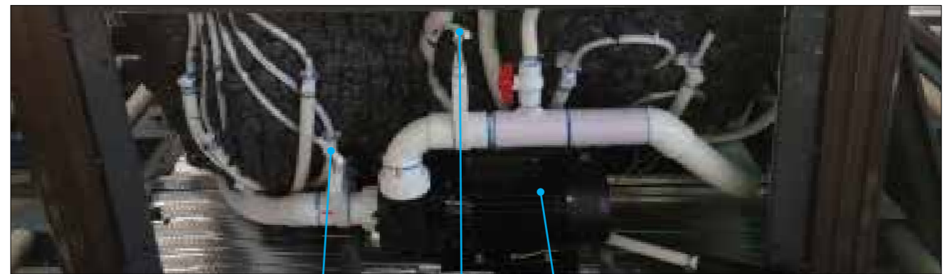
Slice valve Slice valve Pump
