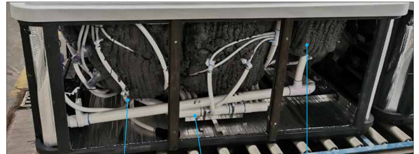
Slice Valve Manifold Black out insulation
