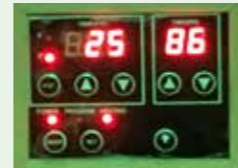
Fig 1. POWER & HEATING lights illuminated to show sauna in operation
